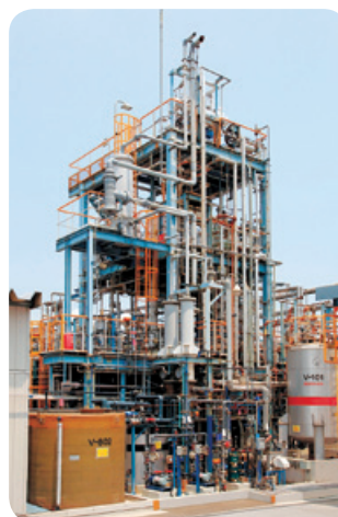
High-purity gas plant
